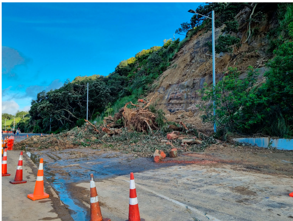
Figure 3. Tamaki Drive land slip after the extreme rainfall event on 27th January 2023. In this photograph, a large tree that fell onto the road had already been partially cleared. This is a major road serving the eastern bays of Auckland and it remained closed for several days.
